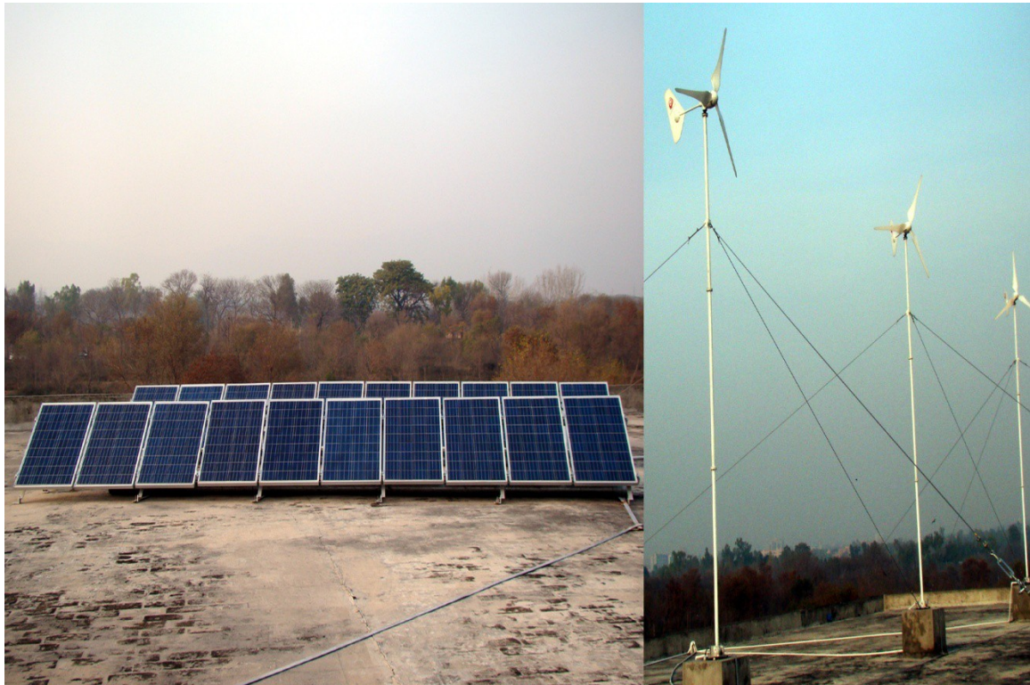
Figure.2: View of Hybrid micro hydro demonstration units installed by Chinese experts at PCRET.
